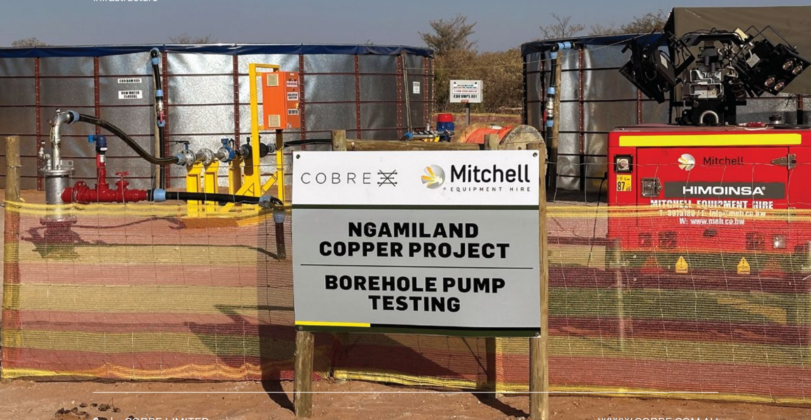
NCP pumping infrastructure
